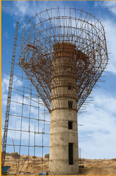
DHA BWP WATER TANK
